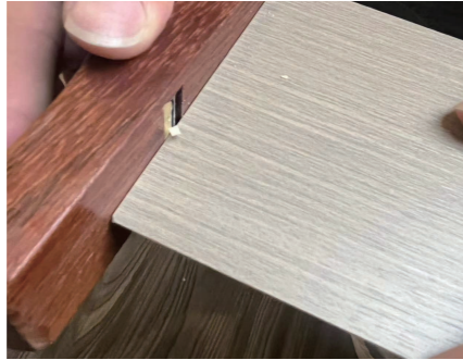
Take out the upper part of the wooden planer with one hand and stabilize the wall panel with the other hand. Pay attention to hand safety
