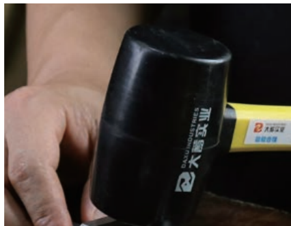
Find the right tapping position The edges and middle of the wall panel need to be tapped
